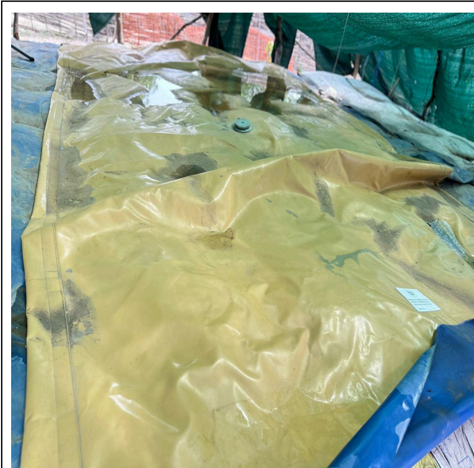
The Majook-Noon PHCC water yard at Majook-Noon boma in Aweng showing the bladder tank which currently non -functional
