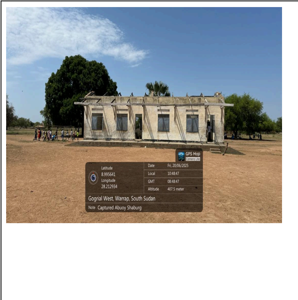
Block of 2-classrooms in Tuele Centre prioritized for renovation in Pan-Nyok Payam of Twic County
