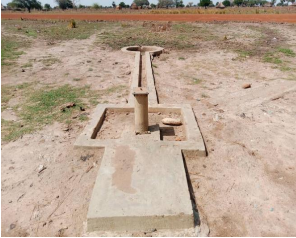
Existing but non-functional community boreholes
