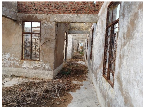
Abandoned Secondary School and Primary schools respectively at Pakur ,Rubkona. © IOM 20 th June 2024
