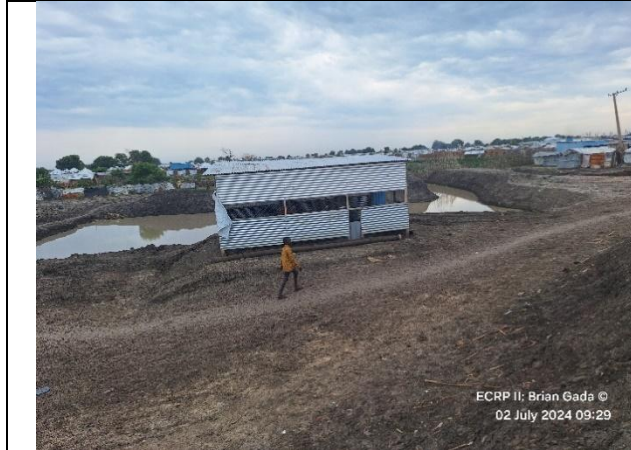
A central drainage water collection point equipped with a pumping station managed by IOM working with local community
